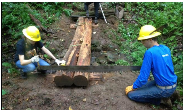
Crew members Zoey and Matthan cut kerfs along the walking surface of the footbridge.
