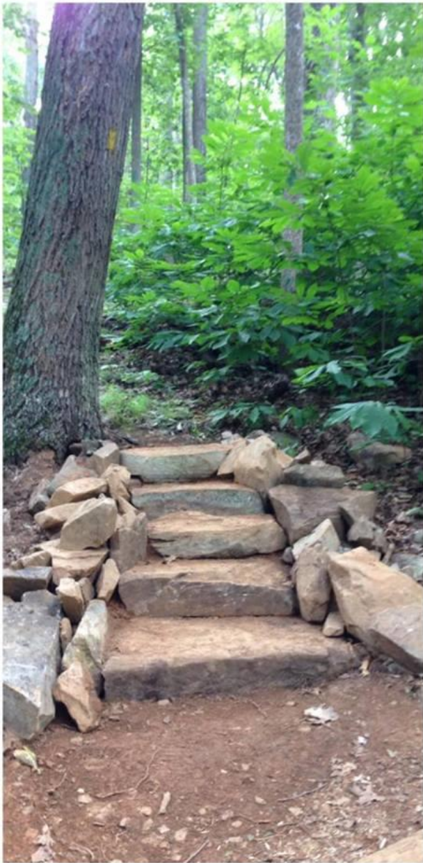
These five rock stairs were completed in a day and a half of work. This was one of the final projects, and the members themselves took lead with the design and work.
